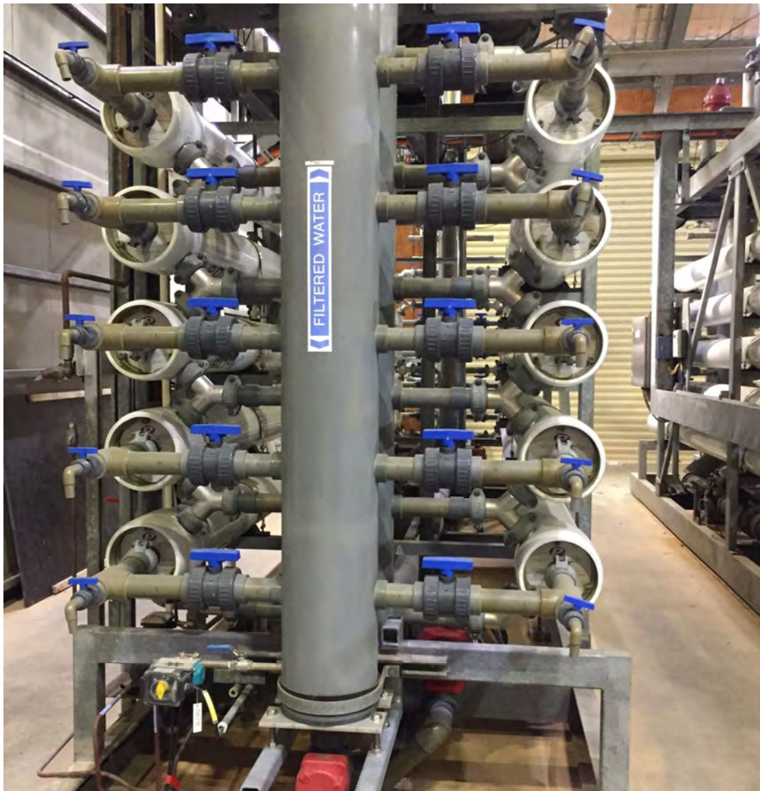
Plate 1: Membrane filtration chambers at Emigrant Creek Dam WTP, October 2019.
